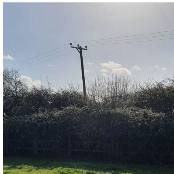
Fig 1.93 - Overhead lines crossing site
